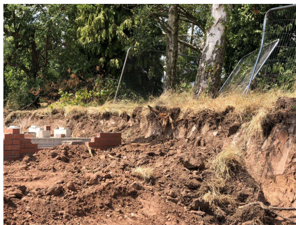
Figure 2: unacceptable tree protection and site standards, with major structural root damage.
